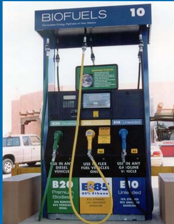
Courtesy of DOE/NREL, Credit - Charles Bensinger and Renewable Energy Partners of New Mexico
